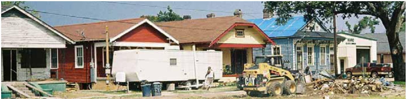
Much repair work remains and a team of STM parishioners is preparing for their trip to help out in February, 2007.
