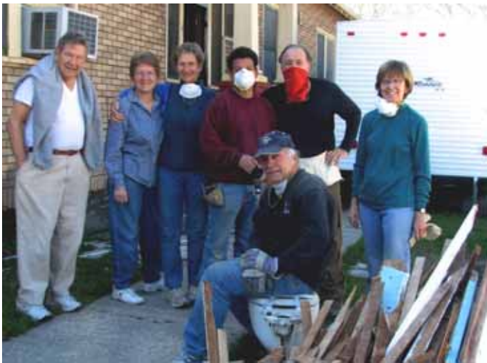
Garmane's team took a moment to pose beside FEMA trailer before clearing debris and prepping this house for new plumbing.
