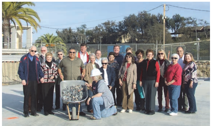
Parishioners and staff members gathered to commemorate the placing of the stones with family names in the foundation of our permanent church.
