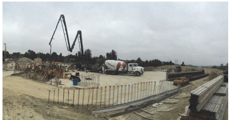
Another major concrete pour on Wednesday, February 19. There was a steady stream of trucks all morning!
